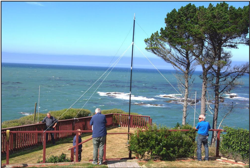
Antenna erection at Moeraki - Paul Aronsen left, Peter Mott (front back to camera), Bill Marsh (right), Paul Ormandy (second from left).
