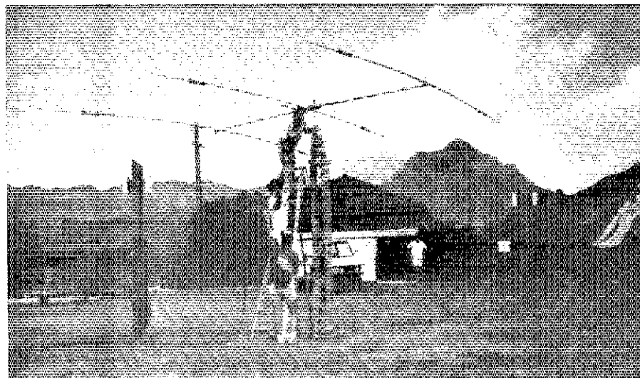
Untangling the coax from the guy wires, these members of the KH6WO FD crew lay the finishing touches on the tribander.
