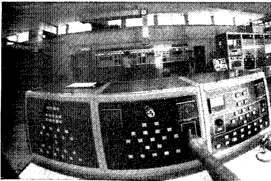
This is the transmitting room for Trans World Radio's facility on Bonaire in the Netherlands Antilles.
