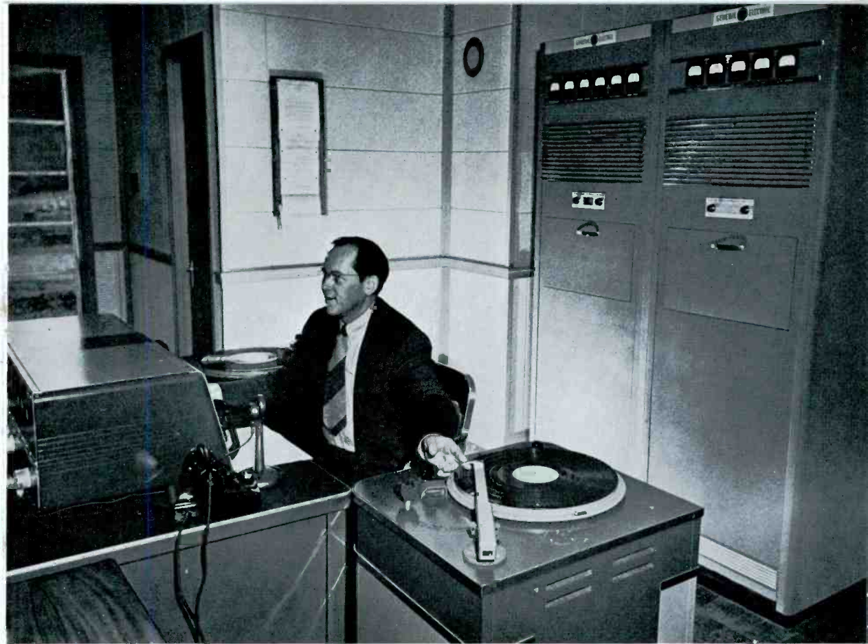
WELLE S. HOAG, W47A CHIEF ENGINEER, WATCHES FOR A SIGNAL FROM THE STUDIO. NOTE THE COMPACT "ARM'S LENGTH" ARRANGEMENT OF CONSOLE AND TURNTABLES
