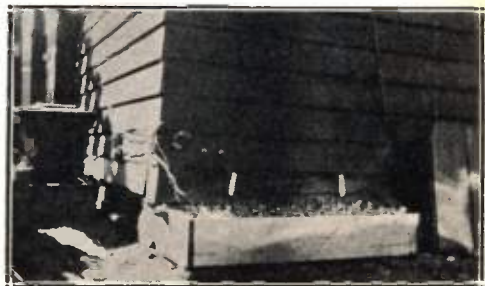
Typical Chemical Rectifier outside the shack (Note the pole transformer)
