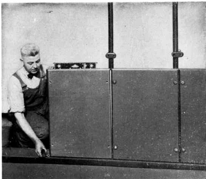
Fig. 24. Spacers are Placed Under the Lower Outside Corner of the Panel When an Opening Appears at the Top
