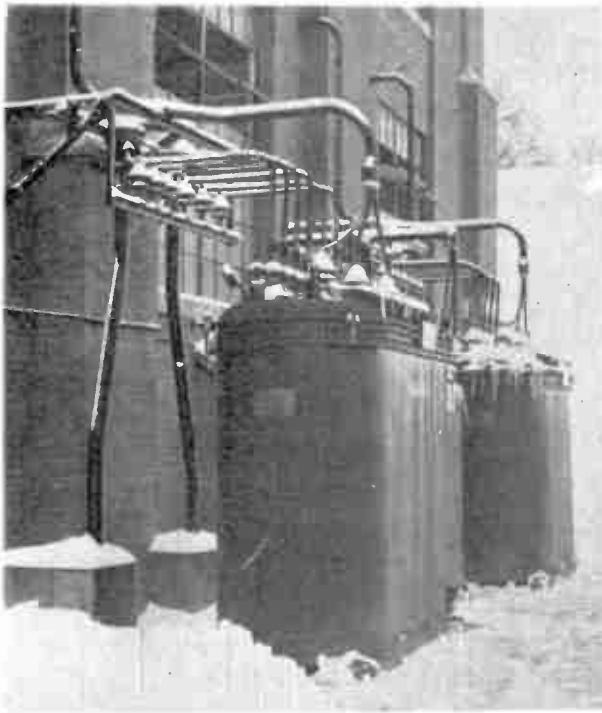
Fig. 47. Outdoor Transformer Installation
