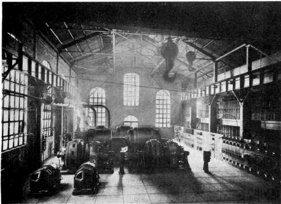
Fig. 16. An Installation Wherein Provision is Made for Future Growth. Note the blank panels and spacious distribution of equipment
