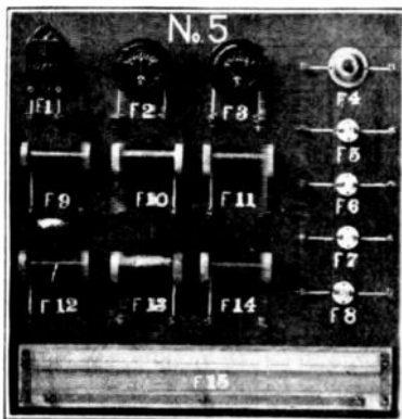
Board No. 5 for electrical testing.
