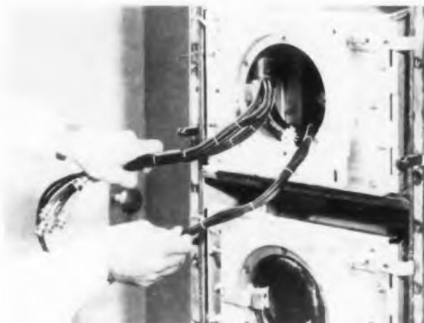
Fig. 8. Use of smaller coaxial cable saved maintenance costs by reducing wear and permitting easier servicing.
