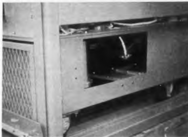
Fig. 13. Entire klystron carriage (left) rides on wheels on NATO "Ace High" 10-kw power amplifiers. Tracks guide entire assembly which can be rolled in or out for maintenance.
