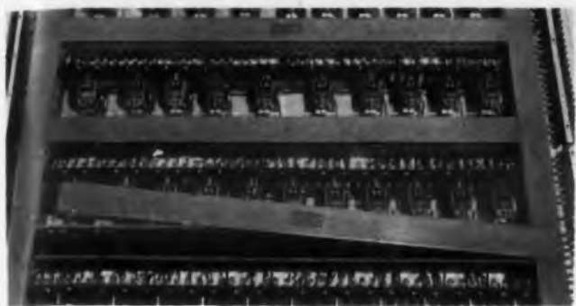
Fig. 4. Taylor Wiring duct allows for neat, easy-to-get-at inter-chassis cabling. Here the duct is used in a large bank of relays.
