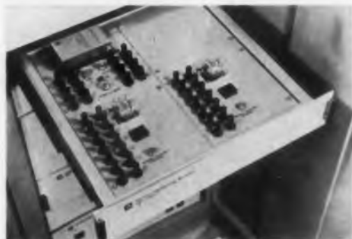
Fig. 22. Centralized test and calibration area, mounted on a pull-out drawer, serves as nerve center in Minneapolis-Honeywell control system.
