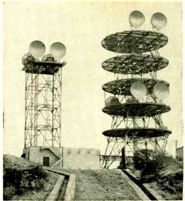
Microwave repeater stations, like this one at Futago Yama, dot the hilltops of the Japanese countryside. Inside the building is a heterodyne repeater.
