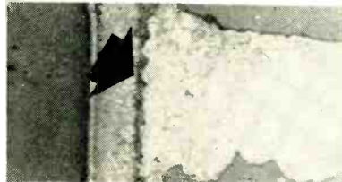
It doesn't take much epoxy to ruin a connection. This discontinuity was caused by smearing of the epoxy during drilling and inadequate cleaning afterward.
