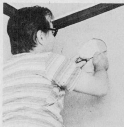
Fig. 3. If the wall is plaster, scribe the outline and then chip out the plaster until the lath is exposed. The lath can be either strips of wood, wire mesh, or plasterboard—a sheetrock-type material with a pattern of large holes into which the plaster locks when dry.
