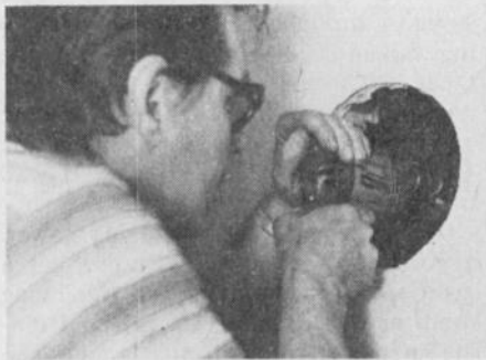
Fig. 5. Remove any insulation between the inner and outer walls and then drill through the exact center of the outer wall. The hole will be the pilot when you're working on the outside. If the wall is masonry or brick use a carbide tipped bit. A standard bit is okay for a frame construction (wood siding).
