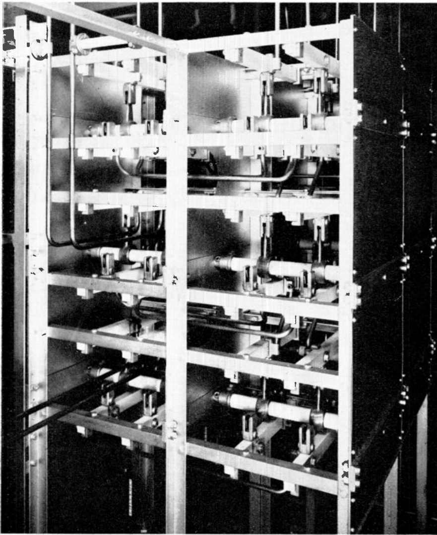
FIG. 8. ANTENNA SWITCHES CONNECT THE THREE 50-KW. TRANSMITTERS TO ANY THREE OF THE THIRTEEN ANTENNAS. POTENTIAL IS 14,000 VOLTS RMS
