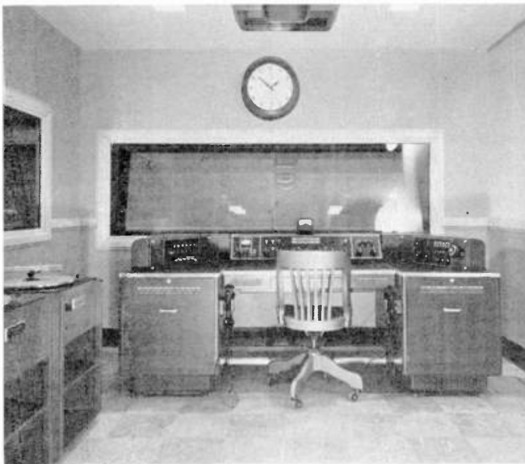
FIG. 7. THIS CONSOLE IS DESIGNED FOR THE CONTROL OF TWO STUDIOS
