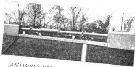
ANDREW FM-AM isolation section with cover removed, revealing two 3/8" FM transmission lines and expansion joints.
