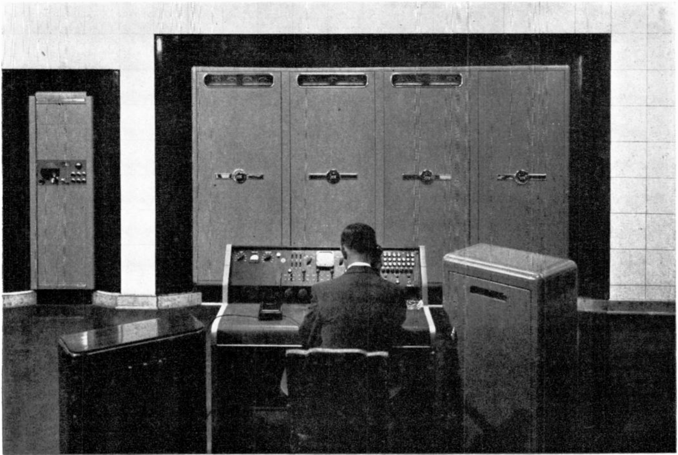
FIG. 1. THE 10-KW. FEDERAL FM TRANSMITTER IS SET INTO THE WALL OF THE ENGINEER'S OFFICE, FACING THE CONSOLE
