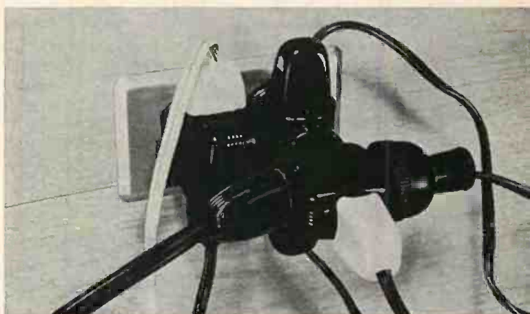
This "rat's nest" is an invitation to danger. You should make use of power outlets on the back of your equipment.
