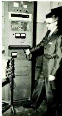
John Radtke, Sherwood's Chief Research Engineer, checks out WKFM's stereo multiplex transmitting equipment.
