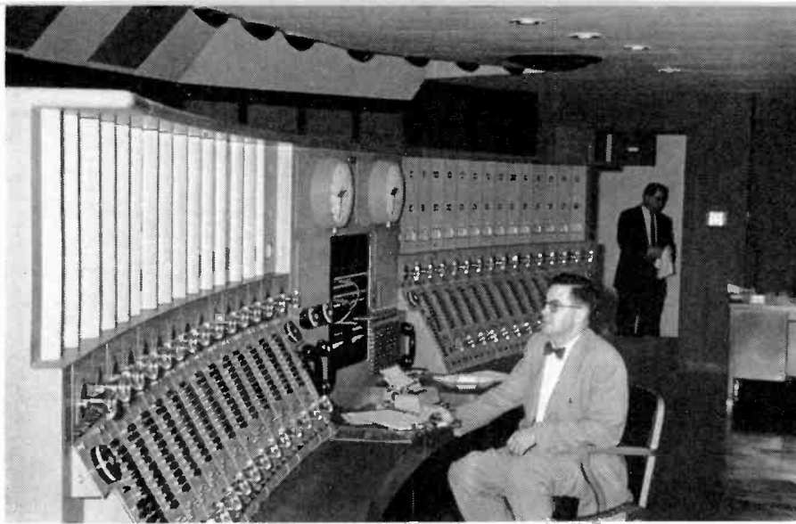
MASTER CONTROL console, Voice of America, has 15 channels on each side of a telephone switchboard and a "remote" switching panel. The swinging feature of each channel indicator and VU meter can be seen in this picture.
