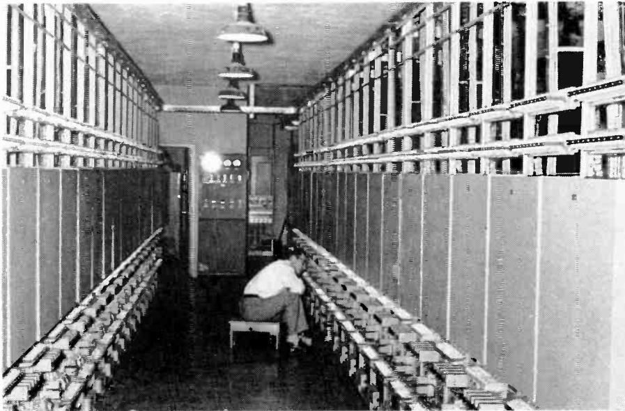
TERMINAL RACKS in the equipment room behind Master Control. The D. C. power supply room is to left, rear.
