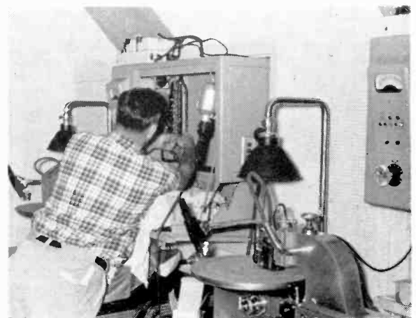
FINISHING TOUCHES being applied to cabinet wiring in one of the recording booths.
