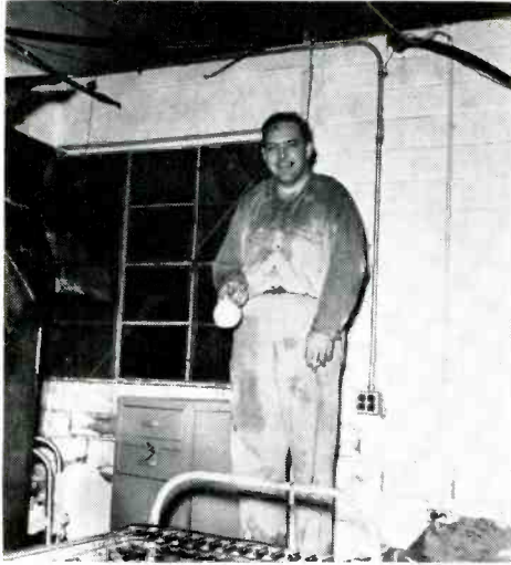
A slightly weather-beaten Chester Rollins stands amid the shambles of the transmitter building with his empty coffee cup. The roof in this portion of the building was blown away by the Oklahoma twister.
