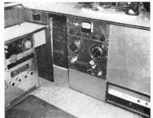
ABOVE: Tape recorders housed under a counter. LEFT: A control console, jack fields, connectors.
