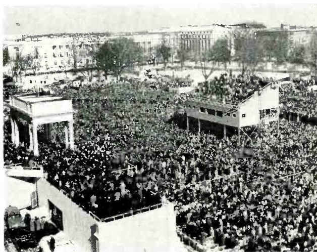
Almost silhouetted against the bare trees of Washington's winter, workmen (top left) put together the framework for a two-tier press box across from the White House. While they worked, the press box at Capitol Plaza was receiving finishing touches. In the 1961 inaugural, the Capitol press box was brimming full (above).
