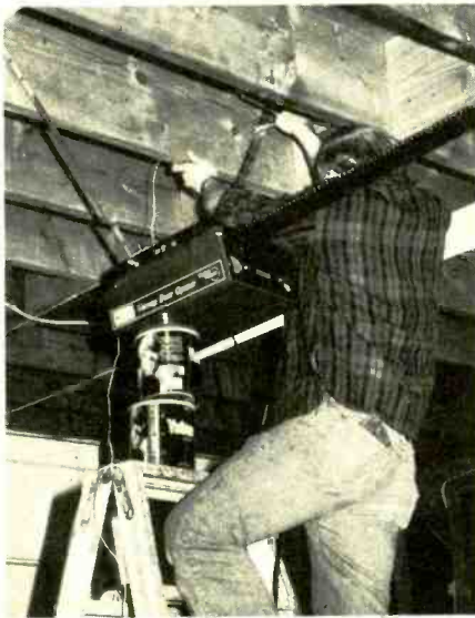
Measure and cut the opener's mounting brackets to size, then secure to opener and joists which nuts and bolts supplied.
