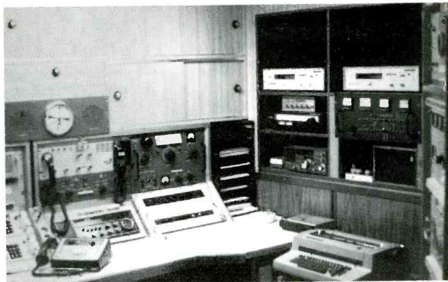
Radio room aboard the M.S. Southward.
