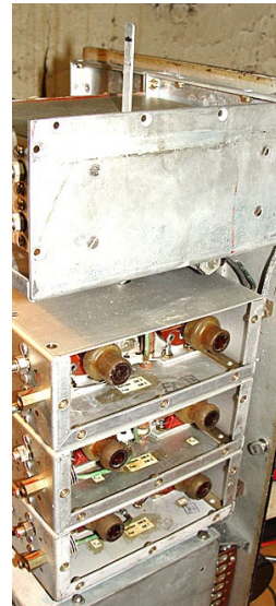
The flat bandswitch actuating rod is visible at top of picture. It is partway along in its journey downward through the switch segments in the three front-end cans.
