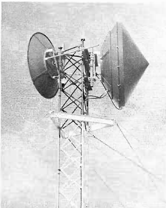
Fig. 23. Typical tower and antenna installation.
