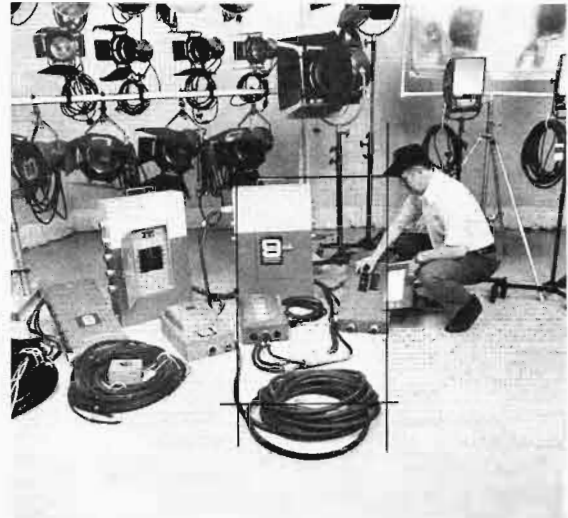
Fig. 42. Lighting circuit breaker panel and disconnects.
