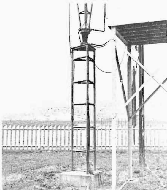
Fig. 41. Example of raising base insulator for flood-water conditions.
