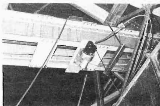
Fig. 25. Power cable hoist at the Chicago Stadium.
