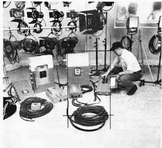
Fig. 42. Lighting circuit breaker panel and disconnects.
