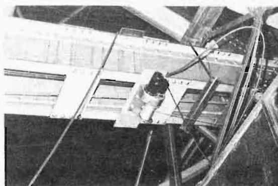
Fig. 25. Power cable hoist at the Chicago Stadium.
