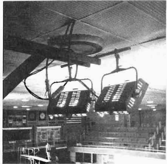
Fig. 39. Swim finals—lamps mounted on outriggers off columns.
