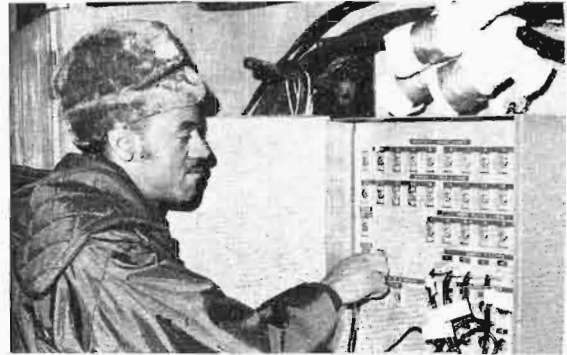
Fig. 52. Audio/video terminal box at mobile unit location, Wrigley Field.
