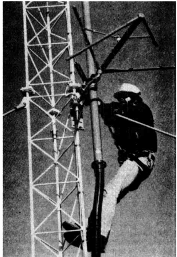
Figure 4.12-20. Rigger finishing electrical tie in box for deicers. Looped stainless steel heaters were factory installed in the four arms, plus one in the feed support boom.
