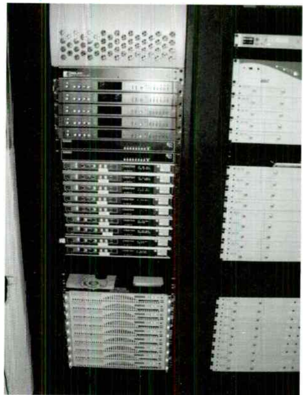
Figure 1. Analog and IBOC tuners, with dedicated webstream monitoring CPUs below and silence monitors at right.
