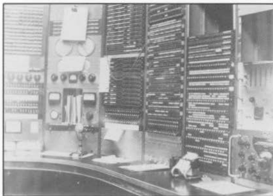
Figure 17. Radio Central's control room in 1960. Notice the absence of cords on the patch bays. RCA's technicians prided themselves on keeping their control rooms neat, so they kept the wiring up to date. Consequently, patching was only necessary for special purposes.
