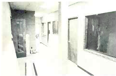
KJR's remodeling plans include new air, news, and production studios, shown under construction.
