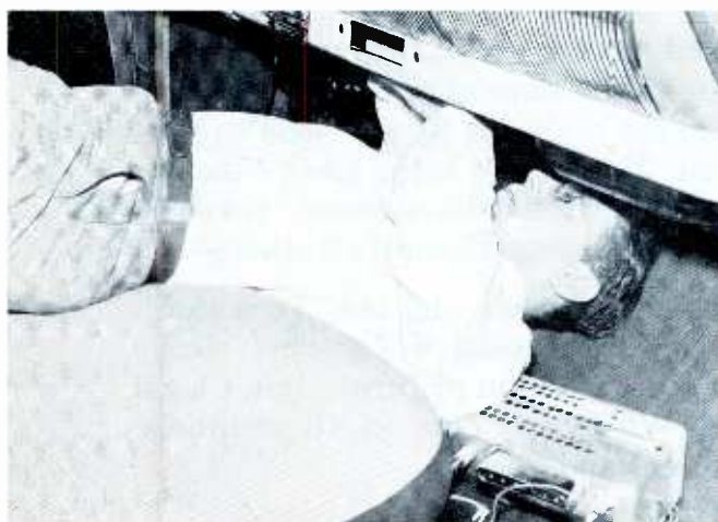
Fig. 6. View of Service Technician Installing Speaker Preparatory to Installing Radio in New Car.
