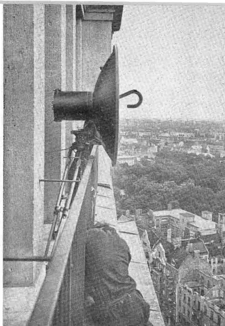
One of the two microwave relay units used in the Berlin telecasts was mounted on the side of the City Hall tower, one of the highest points in the area.
