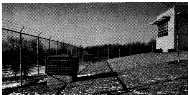
Fig. 7. One of the air intake tunnels which provides filtered air for personnel and equipment.
