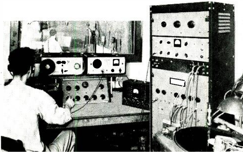
Recording-studio control room. The echo box and its controls are at the top of the rack.
