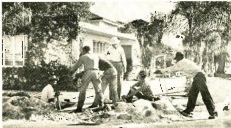
Fos' crew drives pipe across and underneath the street to make way for cable.
