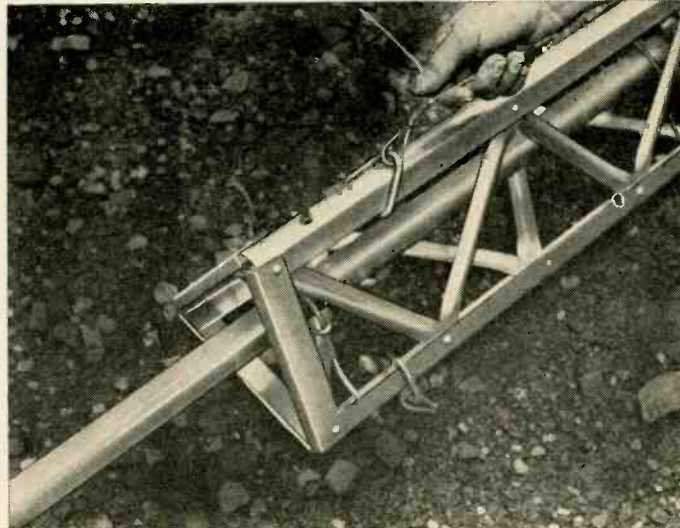
Fig. 7—Triangular guy ring, eye and guy wire attached to top of tower. Thimbles and rings protect guy wire.
