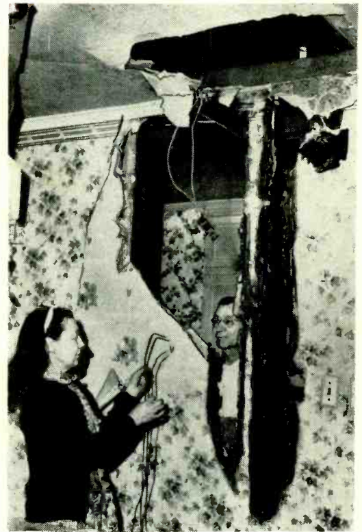
Lightning traveled "down" a TV lead-in and made a new entrance for this kitchen.
