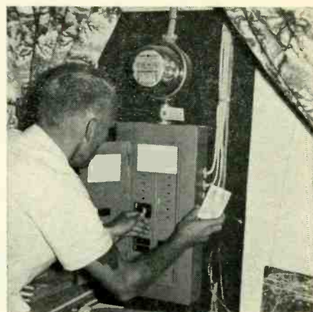
through the breakers . . .
