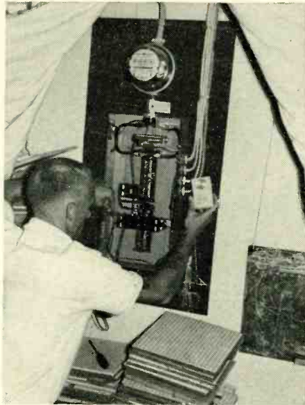
Fig. 4—Transistor portable traces interference on power lines. Be very careful! Pull main breaker or fuses before beginning this test.
