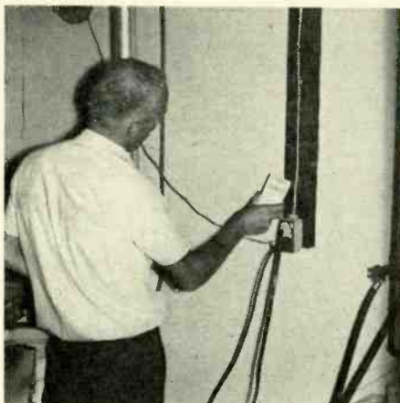
to the outlet box . . .
