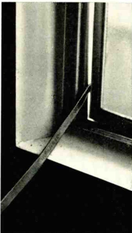
How not to route lead-in; the insulator wears through and the screen won't fit.
