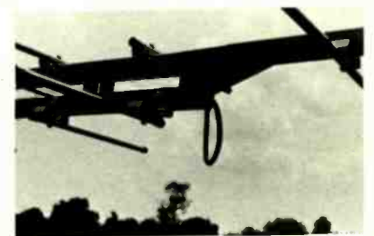
FIG. 13—DRIP LOOP prevents water from running along cable and into connections during a rainstorm.
