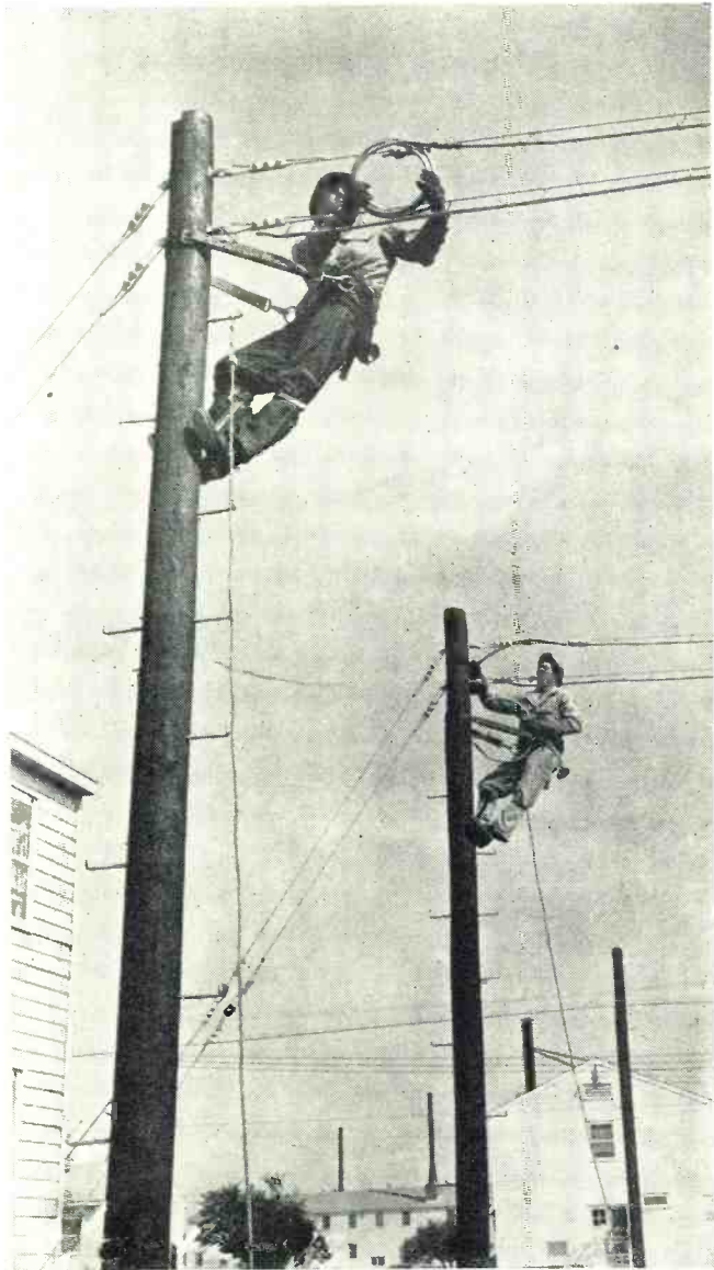
Pole-line construction students of the MSCS school make preparation for splicing cable as part of their training.
