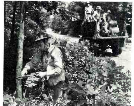
A Signal Corps lineman tying field wire in place prior to stringing.
