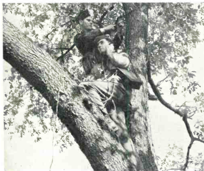
After cable is put fast in position and circuits are ready for test, these men go into action. Note portable phone set.
