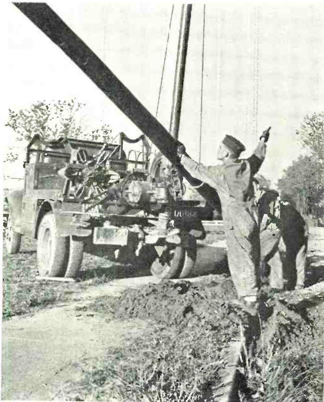
Construction truck equipped with derrick and mechanical "earth borer" used for erection of telephone and telegraph poles by the Signal Corps crews.
