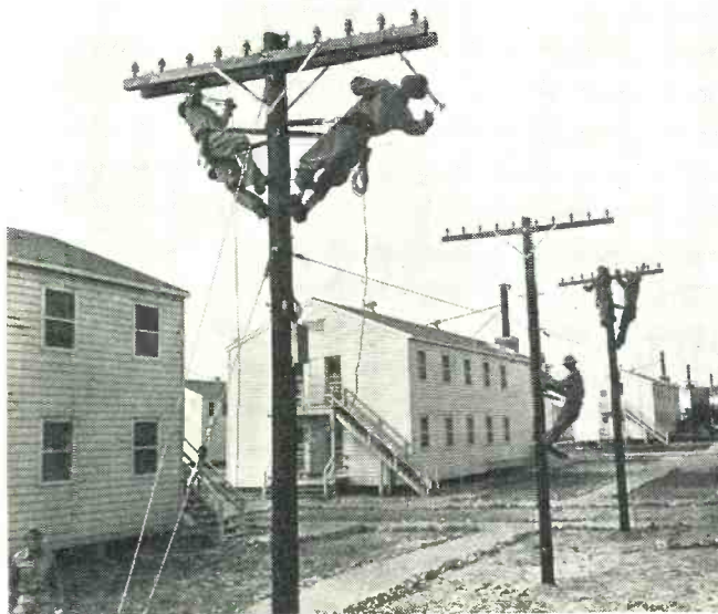
These men are busily engaged in work on combination open wire and cable lead installation. Classrooms in background.
