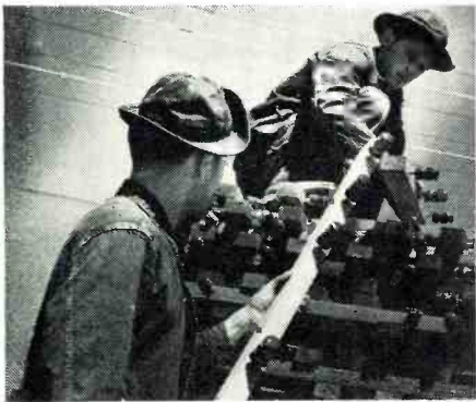
Care must be taken not to damage insulators while stacking crossarms.
