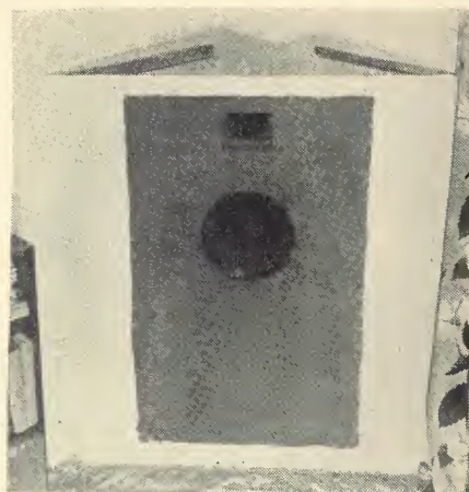
Fig. 3. After the front board is in place, nail a pair of 1 x 1 inch strips to wall to support the top, then paint the area to be covered by the grille cloth with a dark paint so holes do not show through the cloth. Dark green was used by author.
