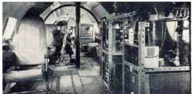
The engineer is orienting one of the directional antennas installed on the plane. Receiving equipment is at the right.
