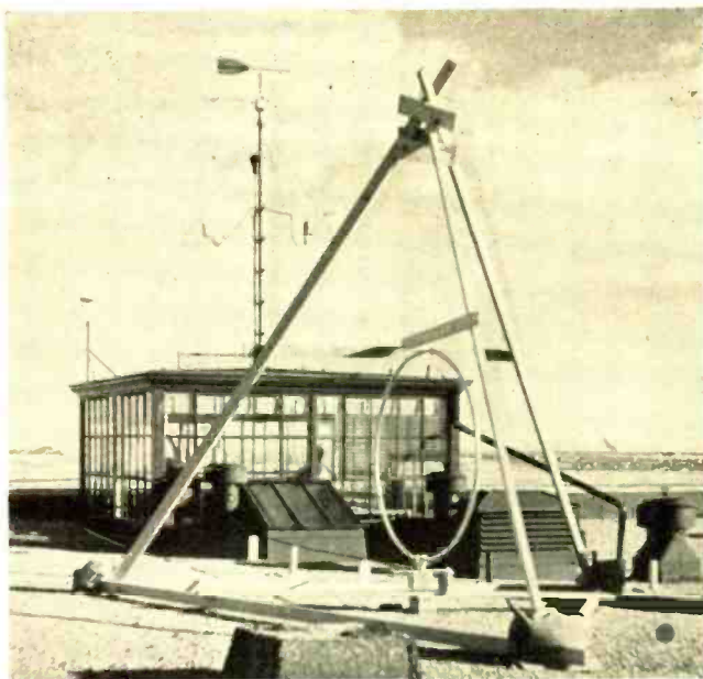
Figure 5. An experimental installation of a static-reducing loop receiving antenna at the Cheyenne ground station.
