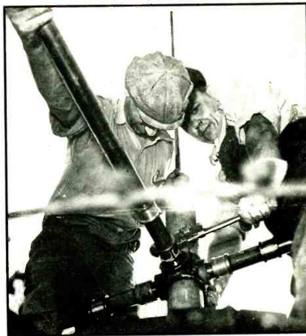
The last of the upper bay radiator elements is fitted into place. Lightning rod rises 5 feet above top of 4-inch supporting pipe. Micarta insulators show at inner ends of radiator elements.
