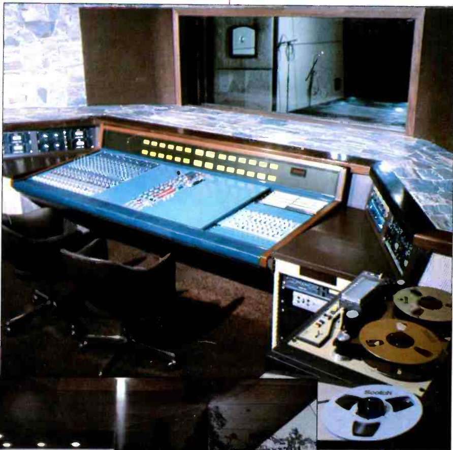
The Master Control Room at Discos de Centro America, Guatemala. Design by Everything Audio.
