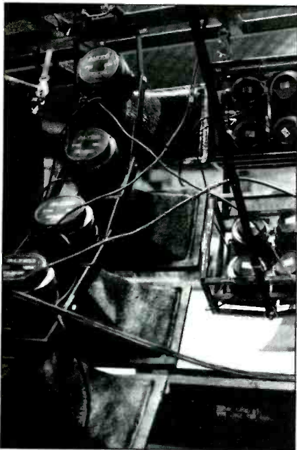
Rear view of Altec horn clusters, showing flexible mount for the Mantaray MR94-8 units.
