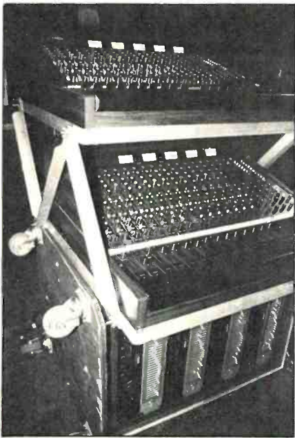
Figure 7: Close-up detail of the collapsible piggy-back stands for M-916 submixers, located on top of crossover rack.
