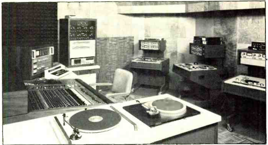
Control room equipment includes MCI/Sony console and tape machines in an LEDE acoustic design.
