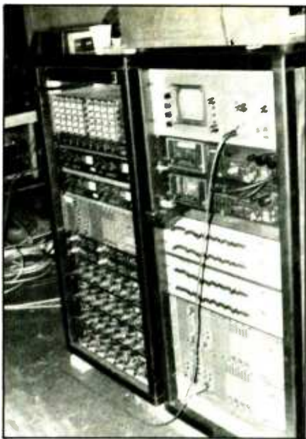
Figure 11: Two of four house electronics racks used on the Styx tour.
