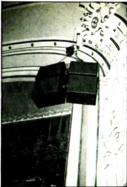
Figure 1: Four Turbosound TMS-3 cabinets are flown by chain hoist per side, to cover high thrust balcony area with direct sound.
