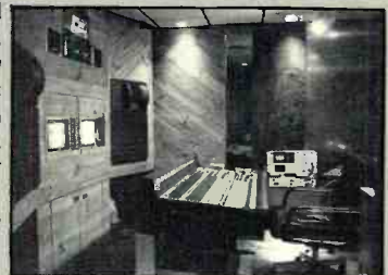
WPCB TV 40 — new audio control room
